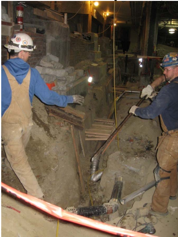
Market Theater Plumbing
