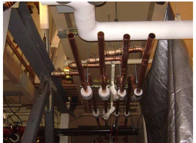
Piping in the Sanitary Market
