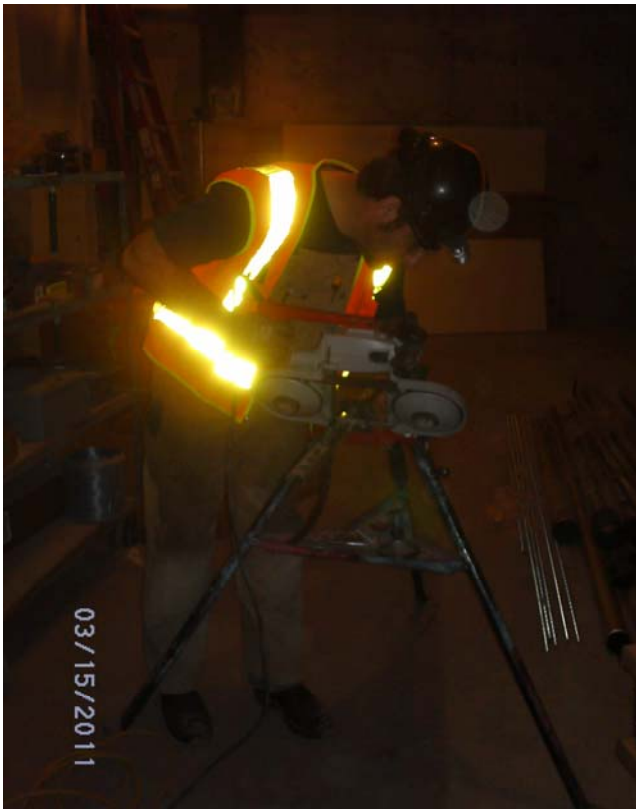
Sanitary Market Electrical Room
