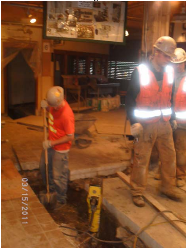
Jack's Fish Underground Plumbing
