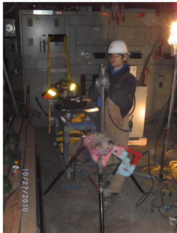
Corner Market Electrical Room
