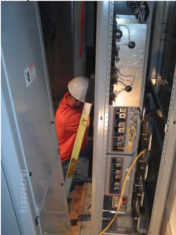
Corner Market Electrical Room
