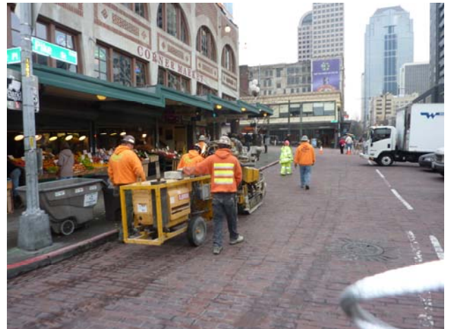
Moving the drill from Corner Market to The Crumpet Shop along Pike Street
